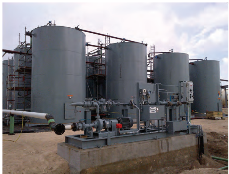
LACT units and storage tanks are manufactured in the Grafton plant
